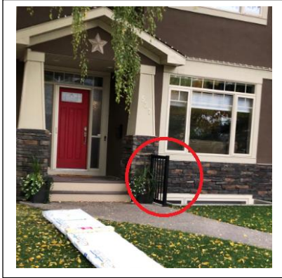
Guard Required Window well adjacent to stairway
